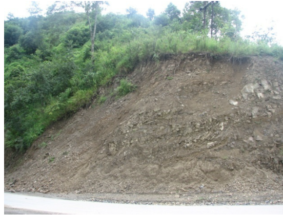
Figure 5 Weak hill slope
